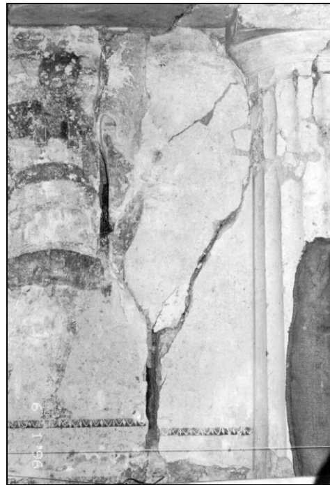
Figure10. Krisis Tomb. The differential settlement caused failures and displacements on the front wall
