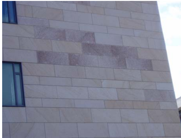
Figure 12. A facade clad with yellowish Chinese granite. Some of the panels are discoloured due to iron bearing minerals has been leached out from the panels and precipitated on the surface.
