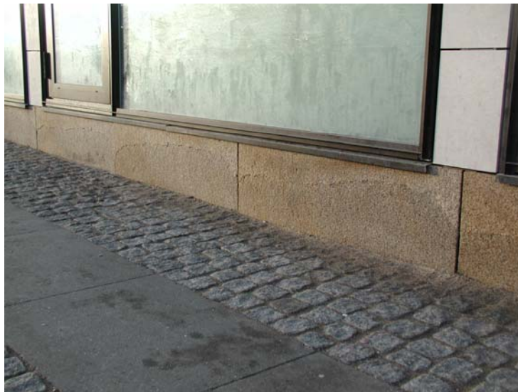
Figure 4. A yellowish, permeable granite with relatively low water saturation coefficient (<80%) showing frost damages (surface spalling) on a building in Copenhagen, Denmark. The stone is however also exposed to de-icing salt.
