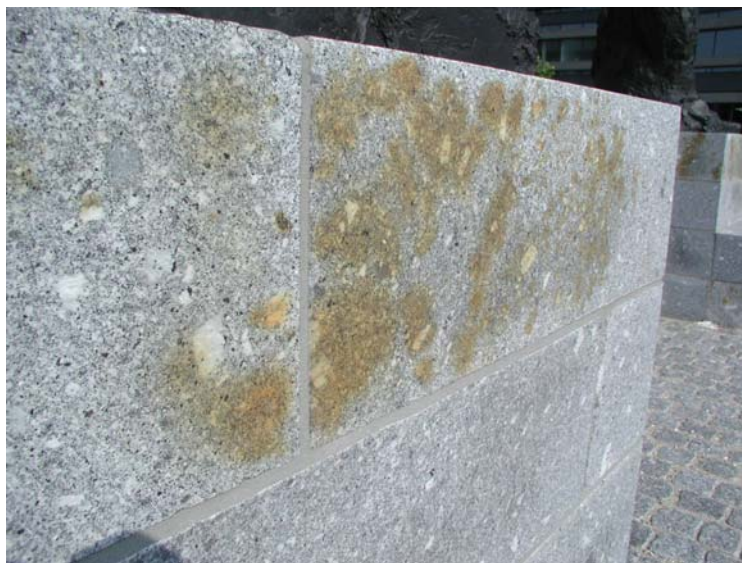
Figure 13. A wall with a magmatic stone type showing rust stains due to the precipitation of iron bearing minerals on the surface.
