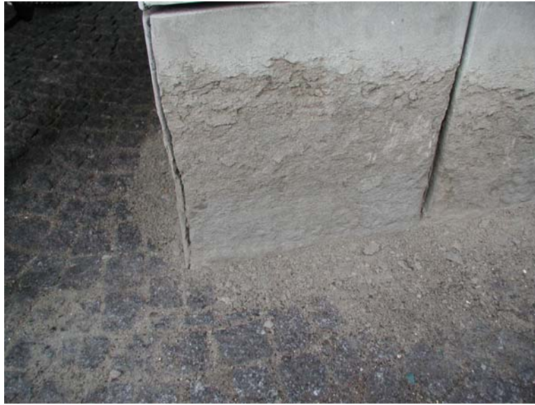
Figure 3. Porous limestone with very high water saturation coefficient (>95%) and severe frost damages (cracking and spalling) on a building facade in Copenhagen, Denmark.
