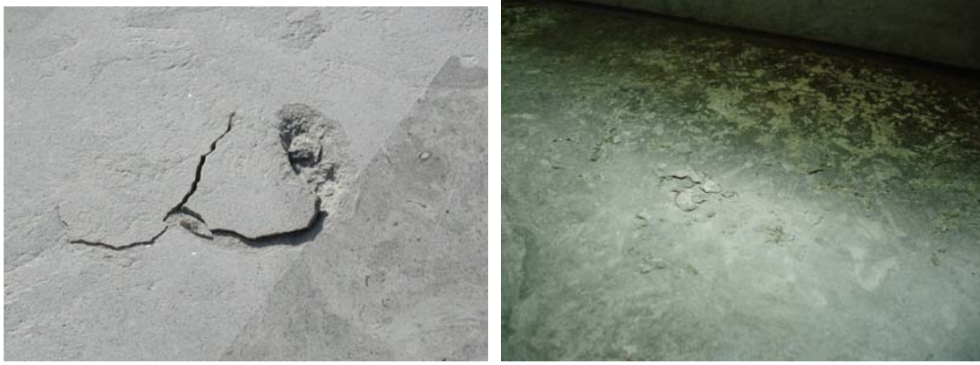
Figure 8. Spalling due to salt crystallisation on the terrace of the National Bank of Denmark.
