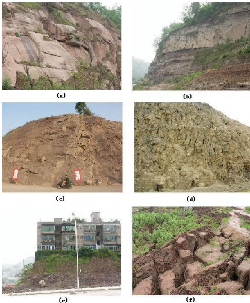
Figure 2. Failure modes for different types of slopes
