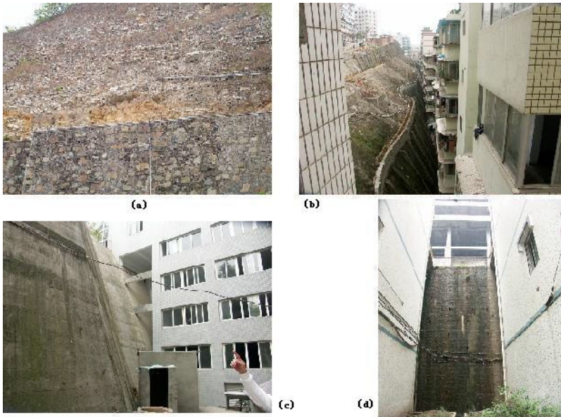
Figure 4. Problems in slope reinforcement
