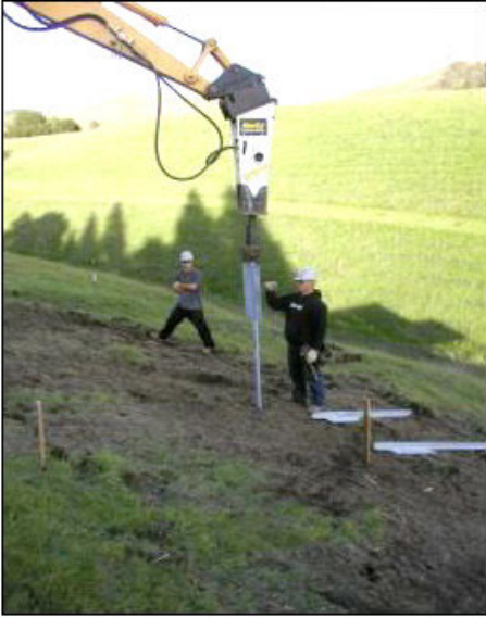
Figure 4. Installation of a plate pile with a modified hoe-ram attachment on an excavator
