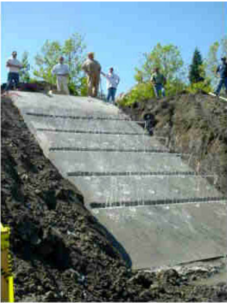
Figure 5. Concrete slab at test site outfitted with an array of plate pile sleeves and subsurface irrigation lines
