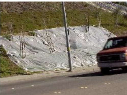
Figure 1. Translational landslide on landscaped slope
