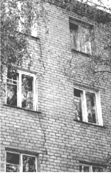
Figure 4. Deformation of house caused by suffosion subsidence in Shchyolkovo, the Moscow region, in 2002
