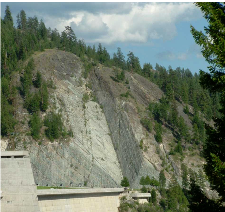
Figure 1. Today's appearance of the mitigated remains of the "Dirty Shame" rock slide of 1970, located at the immediate left abutment of Libby Dam, northwest Montana. This failure occurred during construction and was unanticipated in the course of collection and evaluation of site geologic observations and rock structural data and constitutes a major "lesson learned" in the annals of American engineering geology. The remaining failure trough speaks eloquently for the geologic character of the bounds and properties of the pre-failure rock mass. There were no fatalities. (Image by the author, 2005)
