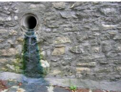
Figure 2. Periodic water overflow in a retaining wall (Veszprém)
