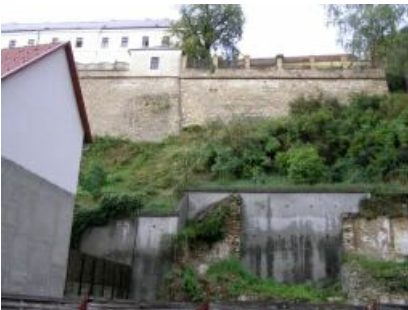
Figure 8. Soaked retaining walls in the castle of Veszprém
