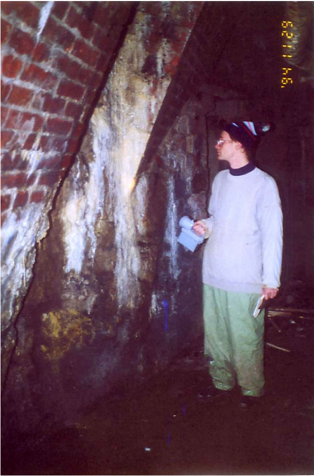
Figure 7. The cave system of the Castle Hill of Buda, water inflow deriving from the defect of public utilities
