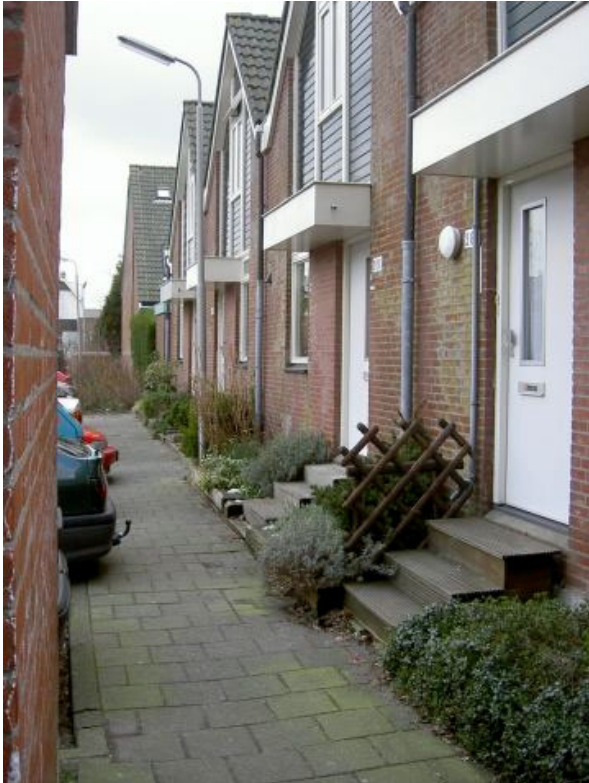
Figure 1. Within ten years after construction, the road settled the height of three steps. Photograph taken in 2004 in the municipality of Boskoop, the Netherlands.
