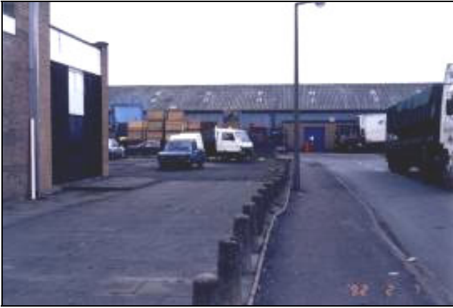
Figure 3. Lateral shear along the outcrop position of the Hollybush Fault, Staffordshire, UK. Note the 0.1 to 0.3 m of shear displacements to the kerbstones, paving slabs and the building's wall.
