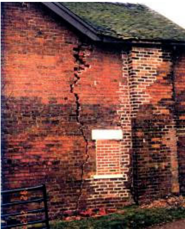
Figure 1. Damage to houses caused by the mining-induced reactivation of the Hopton Fault, Oulton, Staffordshire, UK.
