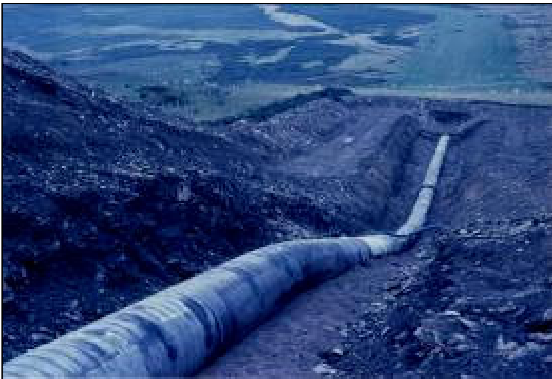
Figure 8. Influence of fault reactivation on gas mains. The Nelson to Dowlais gas main, exposed for strain accumulations and subsidence monitoring where it crossed the Rhos Fault, South Wales, UK.
