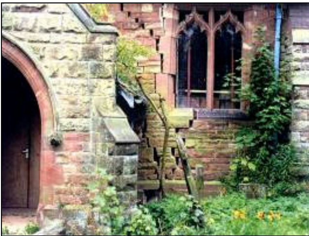
Figure 4. Barlaston church, Staffordshire, UK, was severely damaged by mining induced fault reactivation. The church was partially rebuilt, the tilted and damaged tower and the historical Wedgwood family graves stones repaired.
