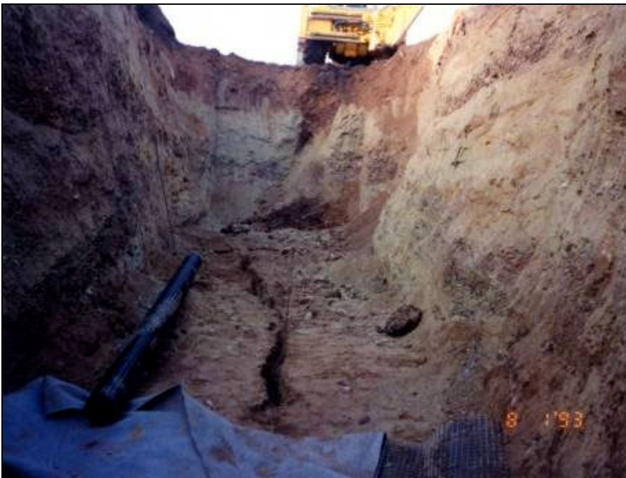
Figure 9. Fissuring associated with the reactivation of a fault, Downes Bank, Staffordshire. This caused disruption to underground communications cables. The fault is exposed in a trench and the ground stabilised using a geotextile mesh and granular fill.
