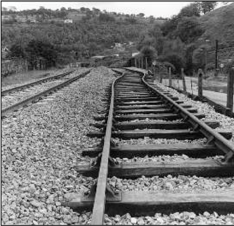
Figure 7. Reactivation of the Kilkenny Fault, South Wales, UK causing severe damage (compression) and buckling to the Cardiff to Taff Merthyr railway tracks.
