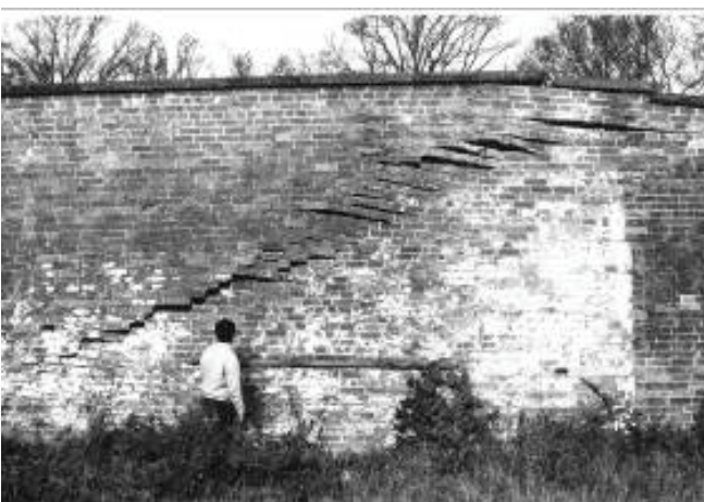
Figure 5. Compression to a 5.0 m high retaining wall, caused by fault reactivation and subsidence, Eastwood Hall, Nottinghamshire, UK.
