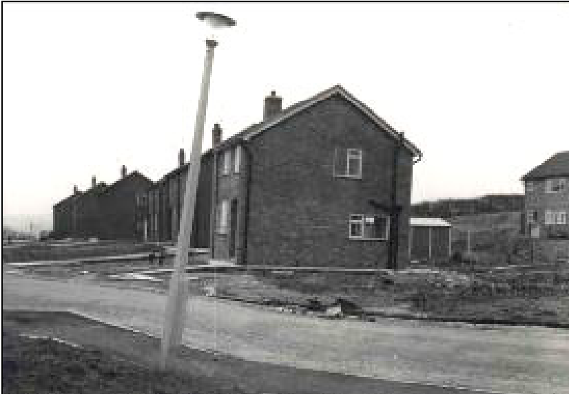
Figure 10. Reactivation of the Apedale Fault, in 1963, causing tilt to a lamp post, (note the vertical string hanging from the lamp post), Knutton, Staffordshire, UK
