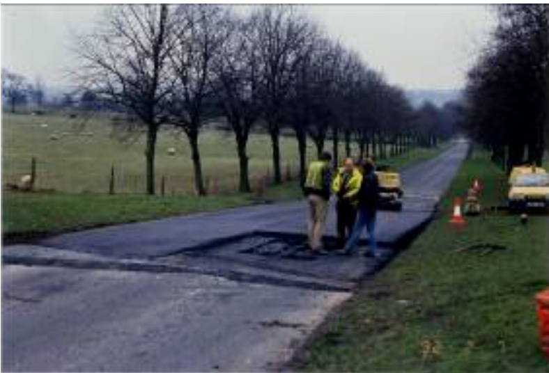
Figure 6. Repairs to Wedgwood Drive, Barlaston, Staffordshire, UK, caused by the reactivation of the Crowcrofts Fault. This generated a scarp at least 1.0 m high and 1.5 km long, during multiple phases of reactivation from the 1960s to 1990s.
